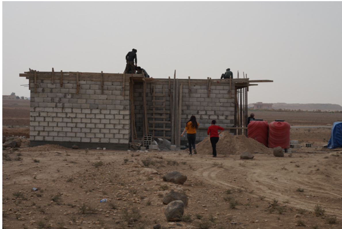
Hasakah new women’s economy project ‘Erd’ - a house is being constructed (now finished!)
